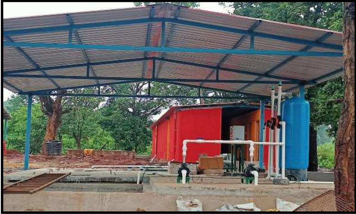
Photo# 7 80 KLD STP Plant at Base Camp
